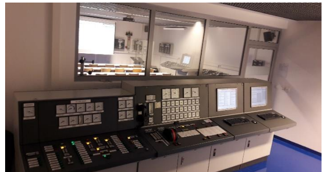
Figure 1. Kongsberg Simulator Control Room
